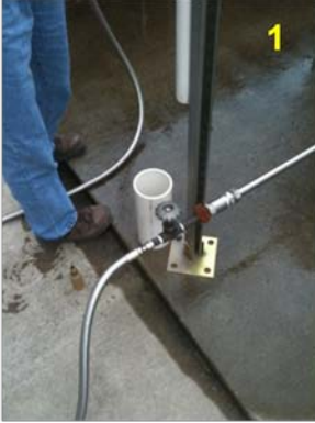
Grey fill station valve
